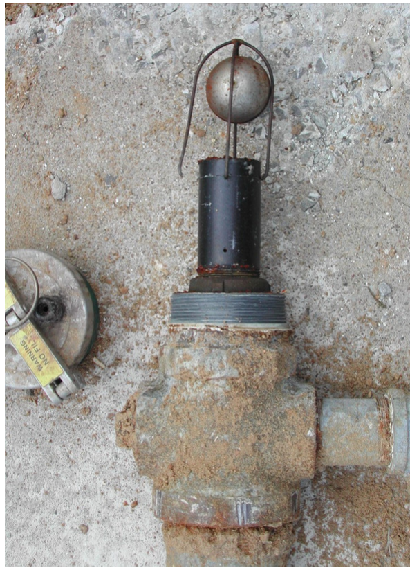
Wire restraining cage is not properly attached.
